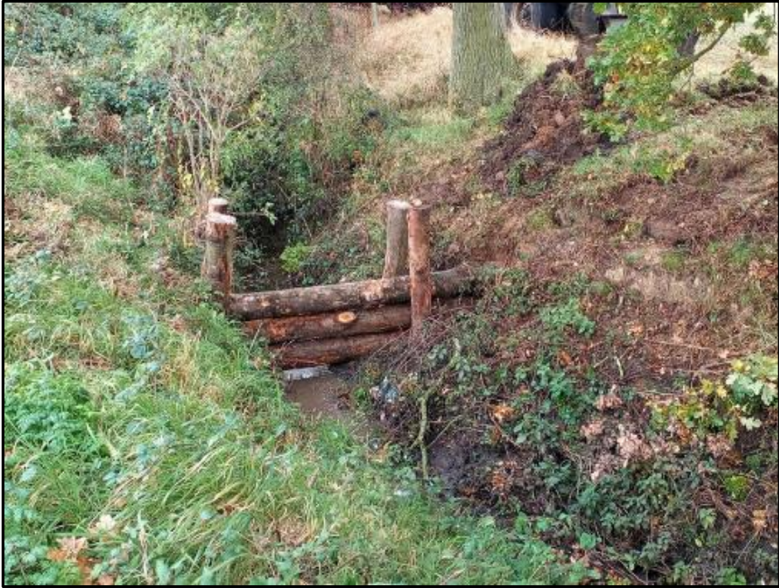
Figure 2. Showing example of field drainage channel leaky dam.
